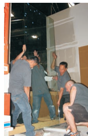
Workers install a glass panel on a case that will display Alaska Native artwork donated by each of the 12 ANCSA Corporations.
