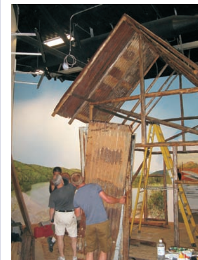
A local crew installs Maudrey and Henry Sommer's smokehouse which was transported from the Yukon River just upriver from Tanana last fall.
